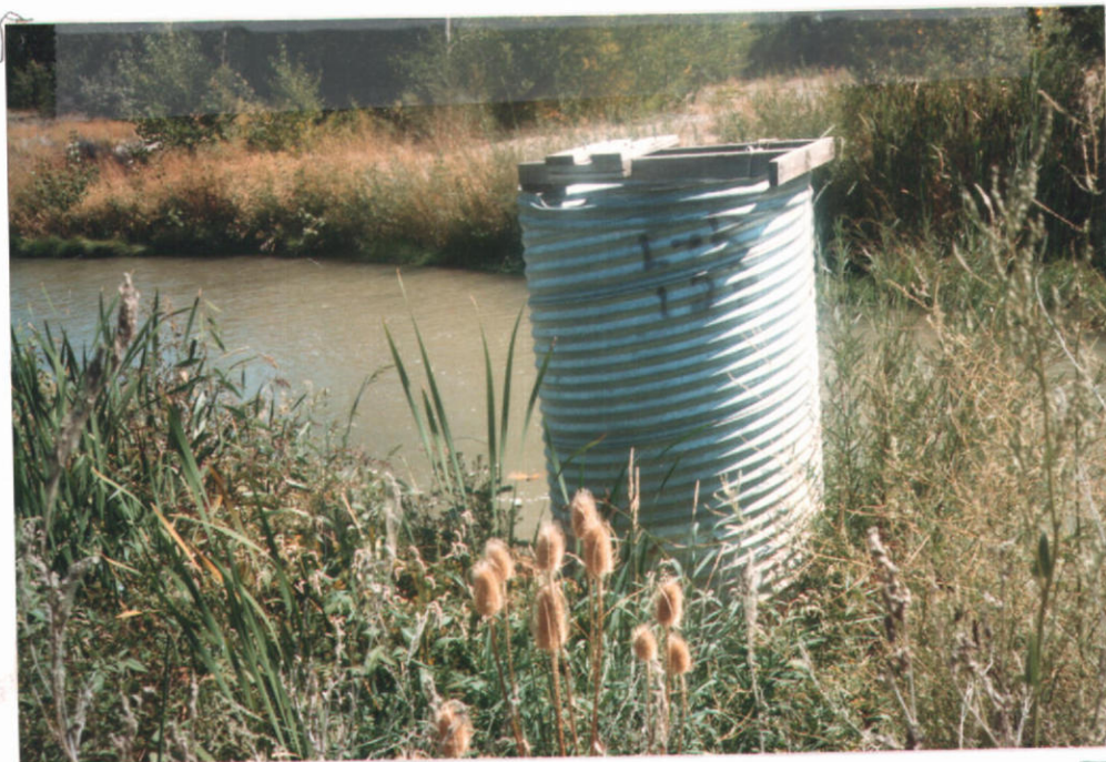
4'x16' CMP sump 7.5HP motor at time of Exam. Time of picture motor being repaired. Success creek.
