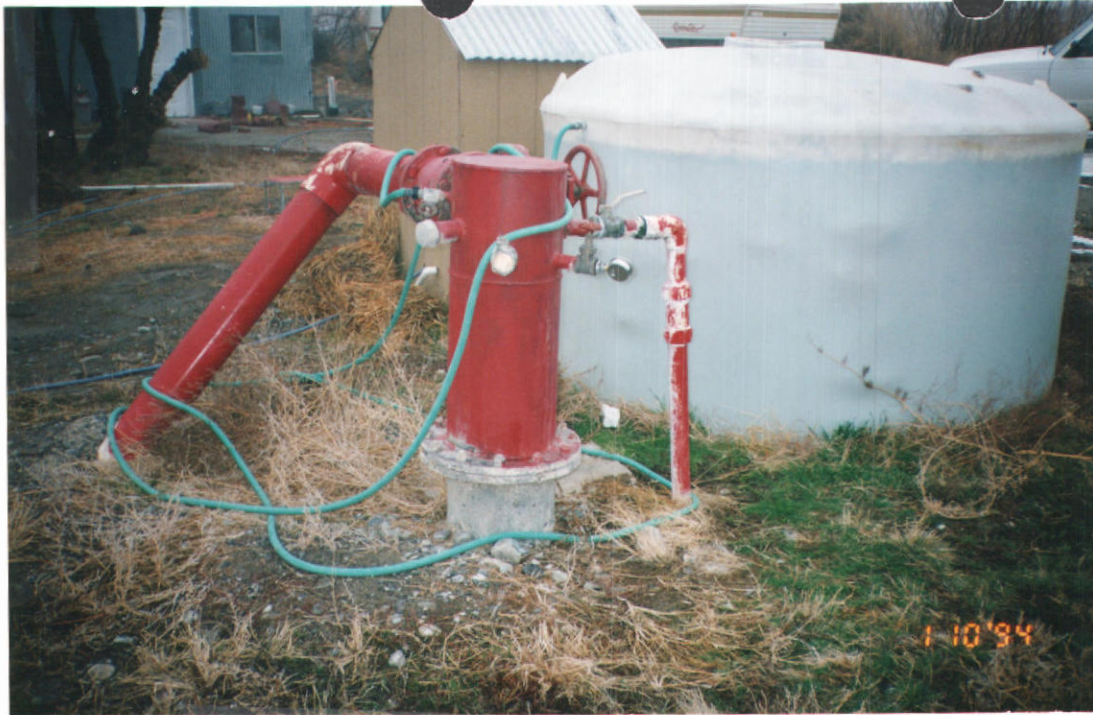
Well (w/ domestic cooling tank)
