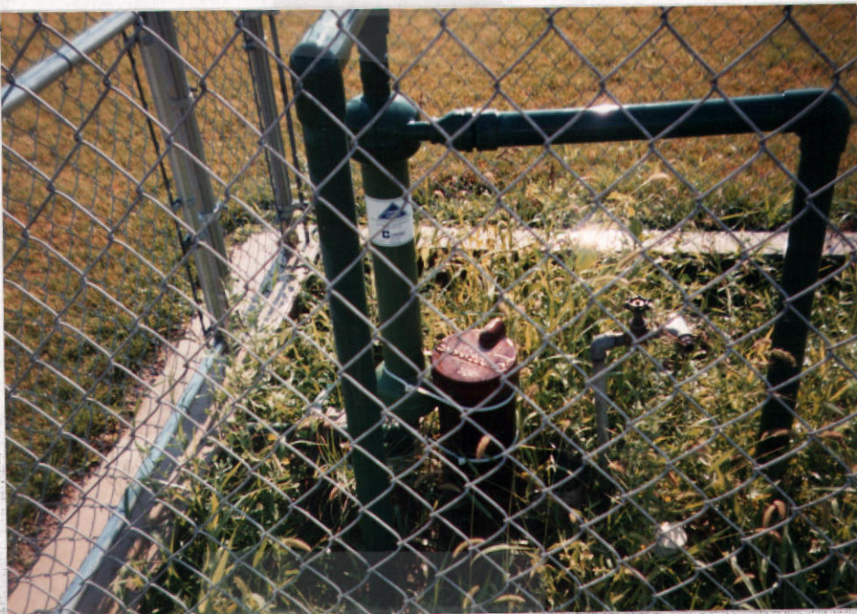
picture of irrigation system. located in the north east corner of the church.
