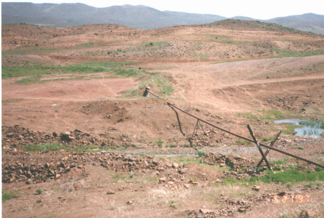
Upper pipe outlet from lower Macks CK Dam. Seepage is from left abutment. below aux. spillway
