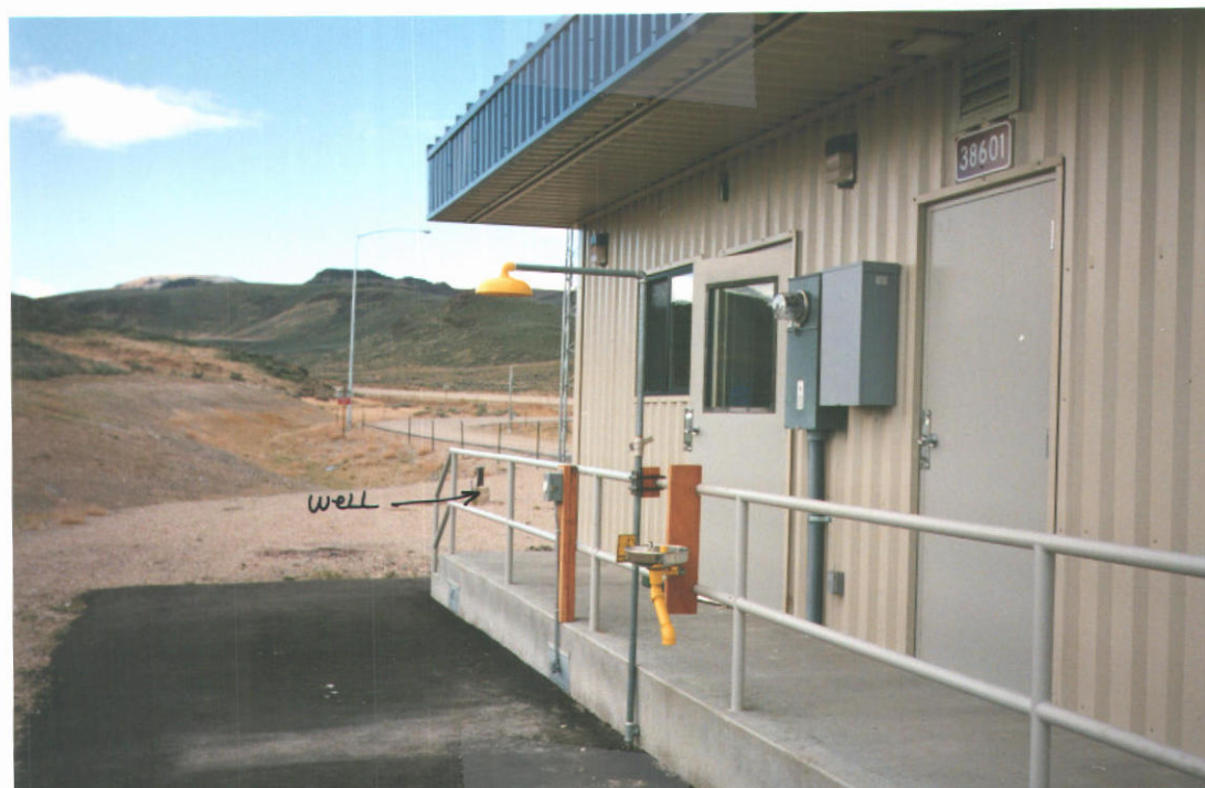
PHOTO THREE- Chemical wash unit in back of office.
