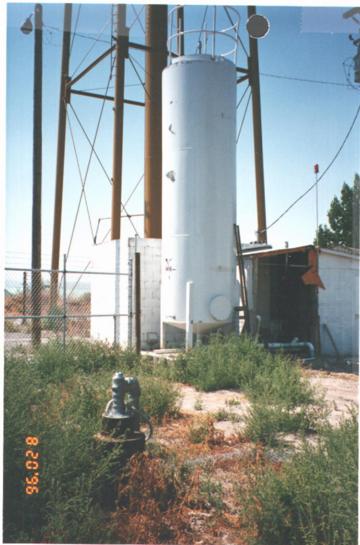
P/D + aeration Tank
