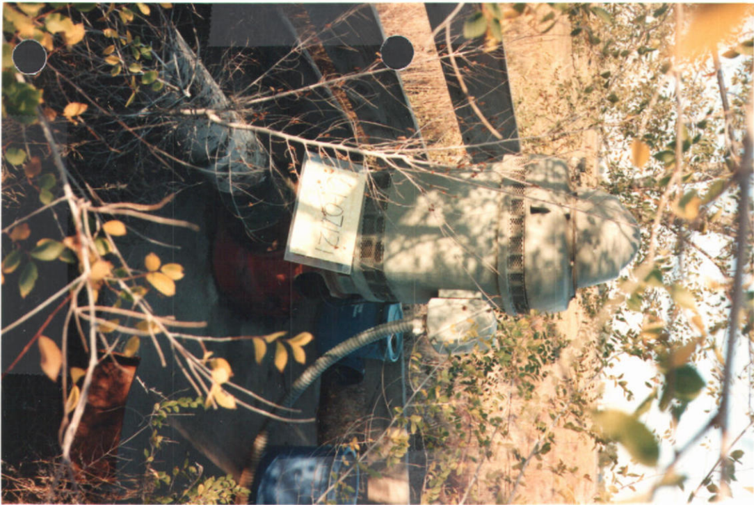
100 HP US ELECTRIC C9981-00-464 84-16095 WELL LINE PUMP 54656 located in NWSE
