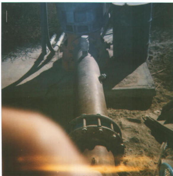
EAST UNDERGROUND 300 HP
