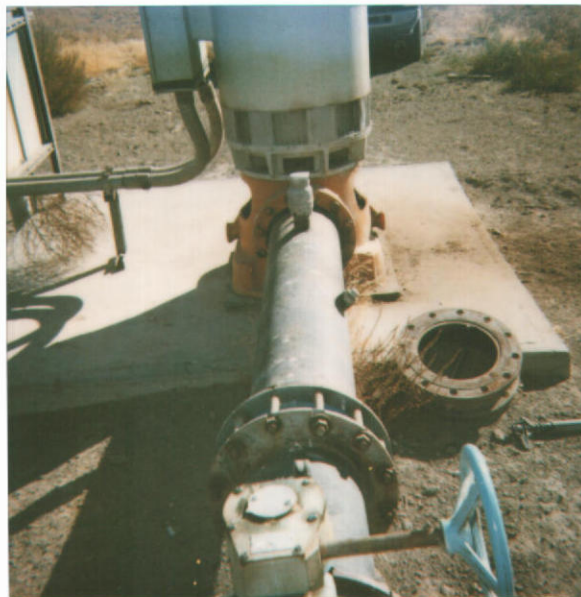
WEST UNDERGROUND 300 HP
