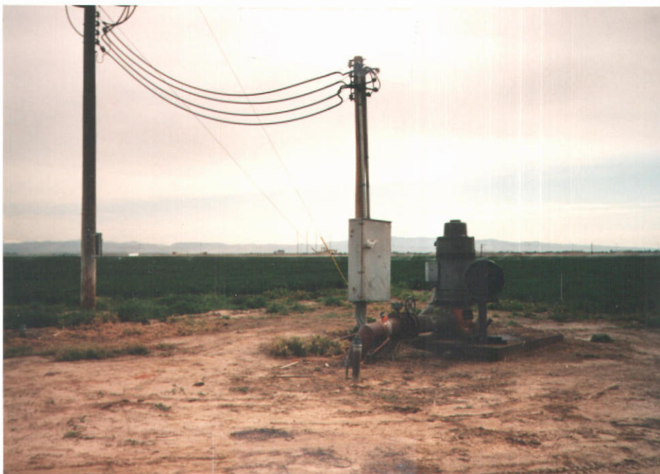
#2 Motor, power source and 10" discharge pipe leading to a 10" buried mainline.
