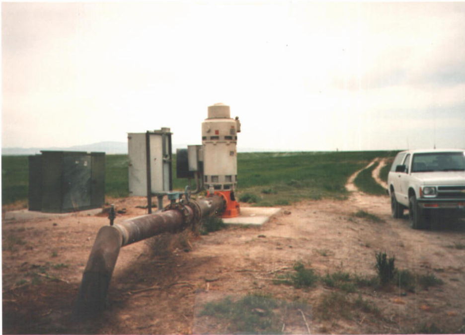
#9. Irrigation well # 3, motor and 10" discharge pipe to buried mainline.
