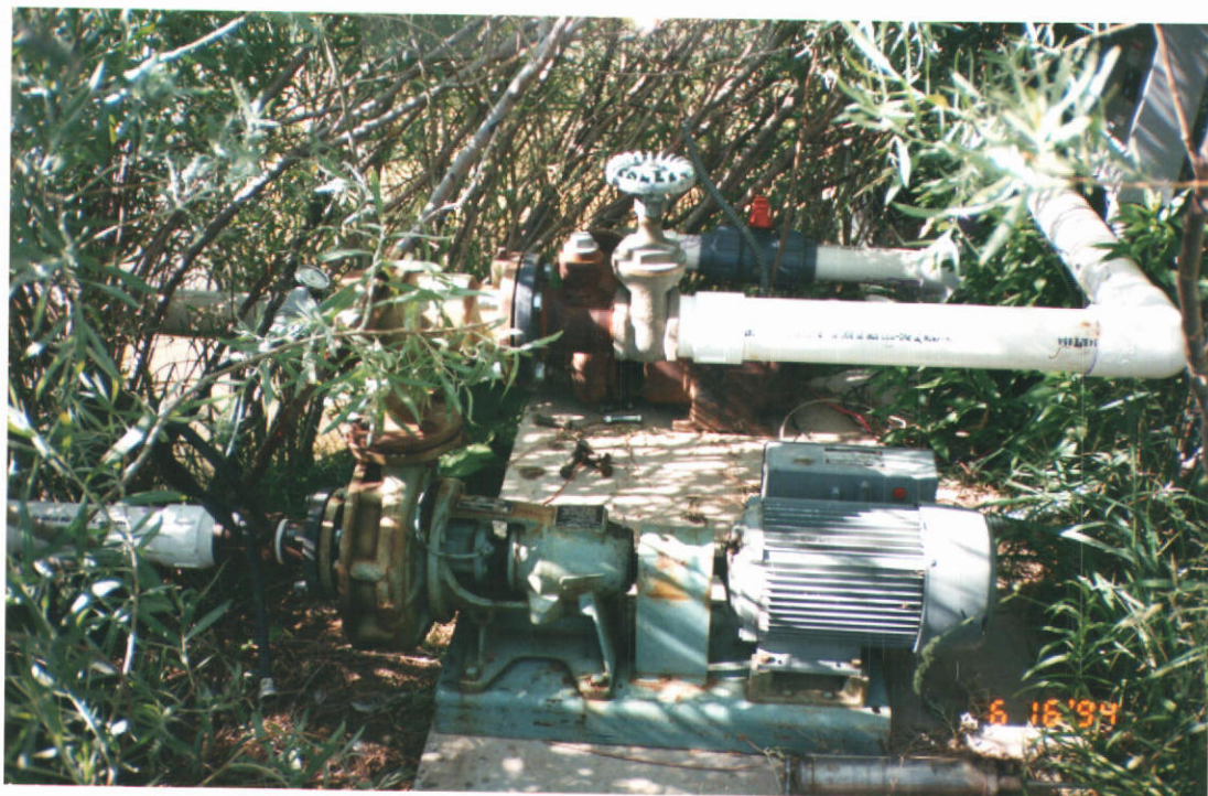
Pump Station - primary (5HP) & backup (3HP) pumps
