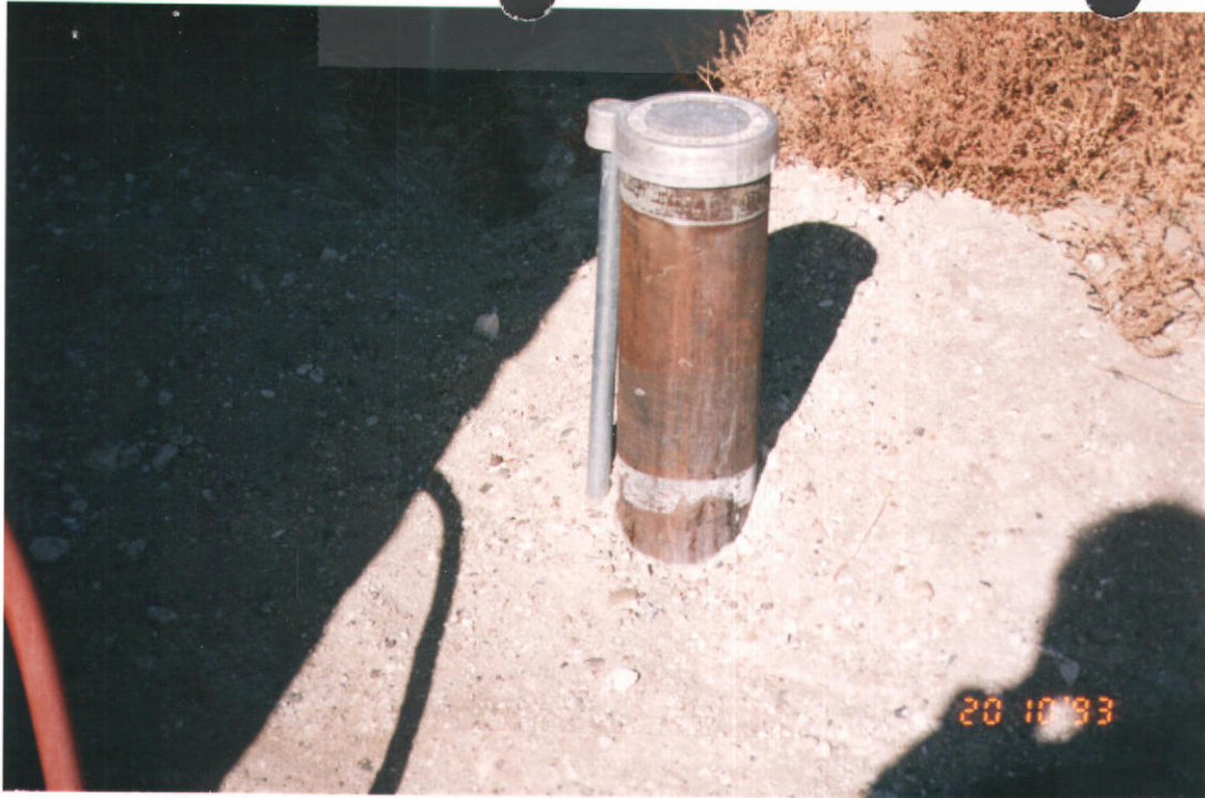
6" well 2.5 HP sub - mersible pump
