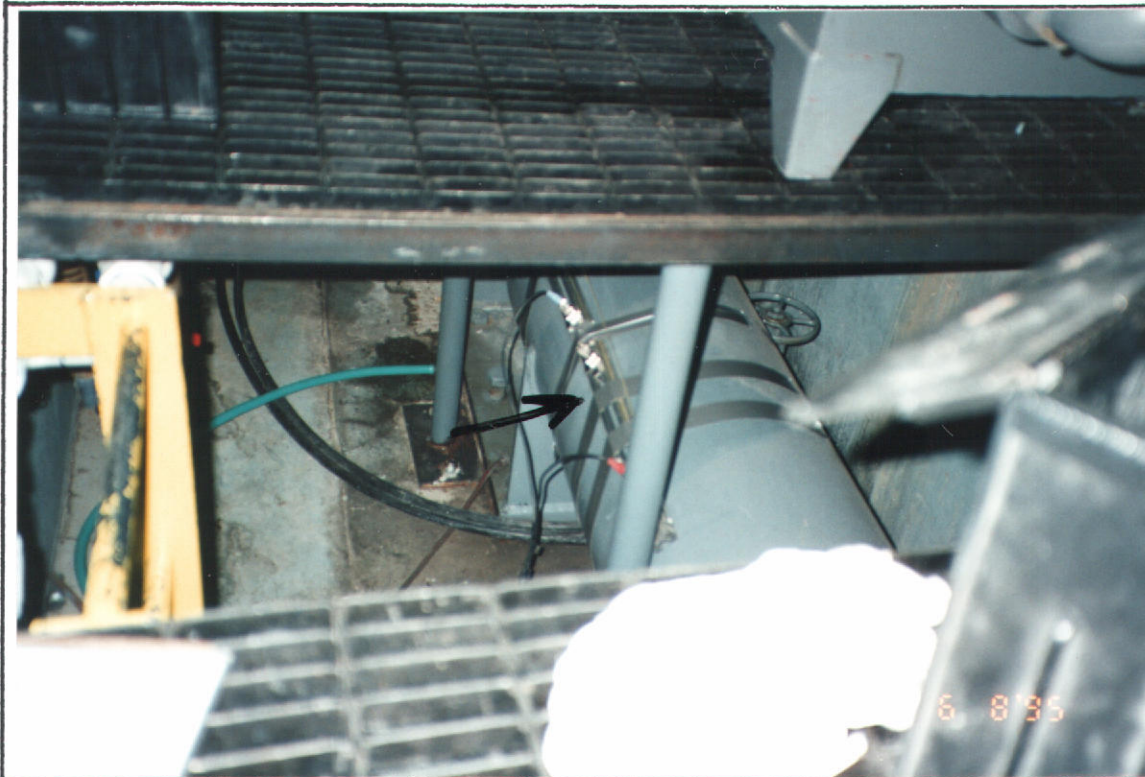
VIEW OF SONIC METER SENSOR ON LOWER TURBINE INPUT
