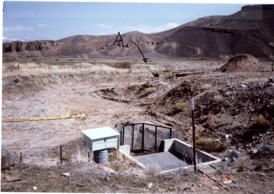
Headgate from ditch "A" entrance appeared closed. Structure in foreground is newly upgraded with screens.
