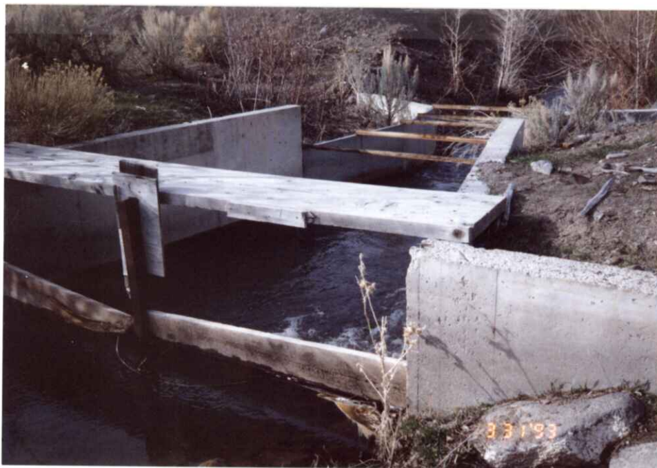
Main diversion from Cottonwood Cr. Note metal parshall flume measuring device.
