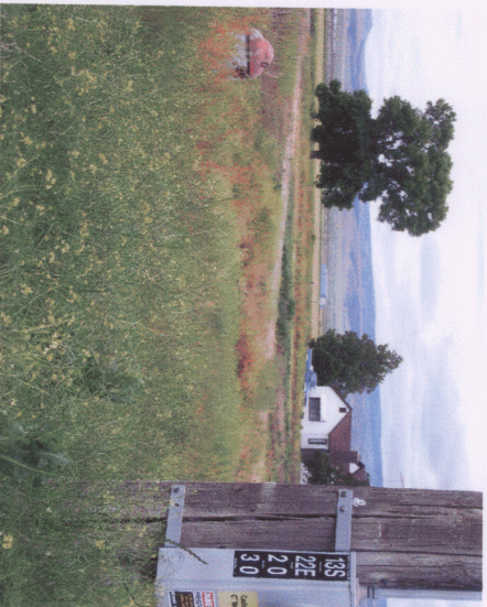
Power Meter (13S22E2030) Supplies Power to South Booster Pump and Well
