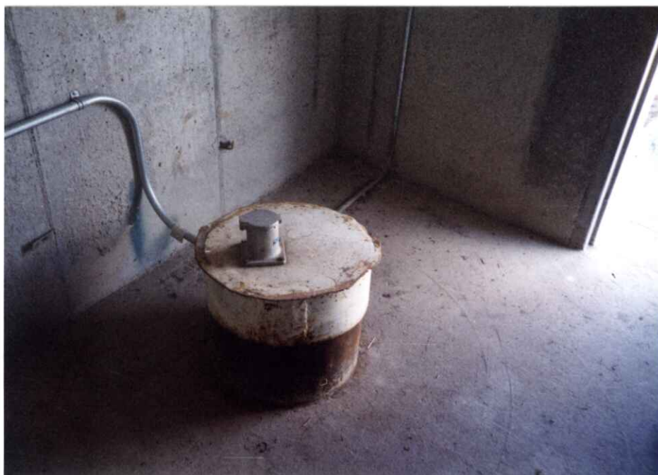
Well inside well house controls at left side of Pretum
