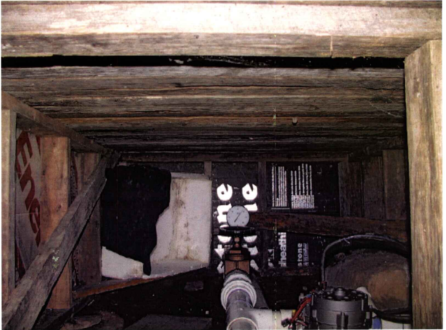
Powerhouse and pressure gage
