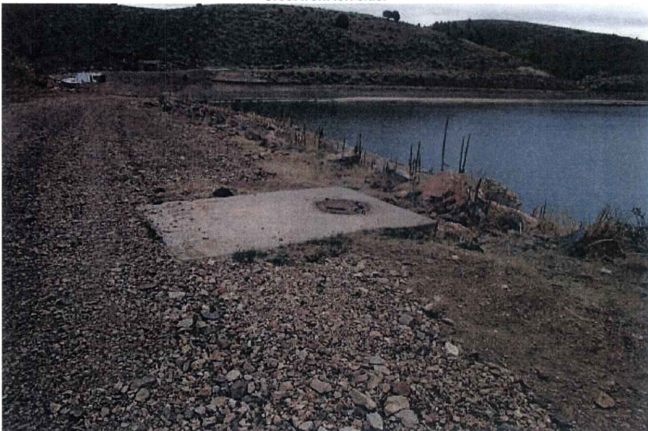
Outlet control man hole.
