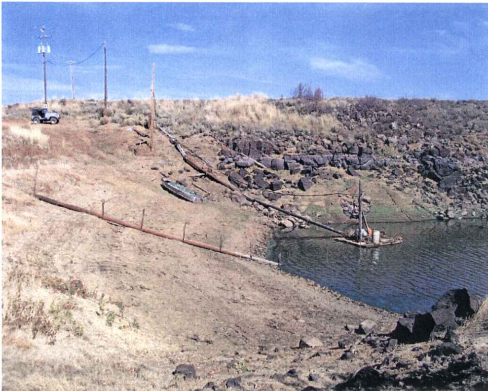
Rhead Reservoir Pumping Plant ( Looking N / NE )
