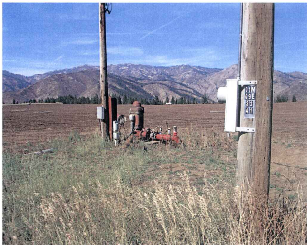
Well #4 – Pole 01N, 09E, 33-41 ( Looking NW )
