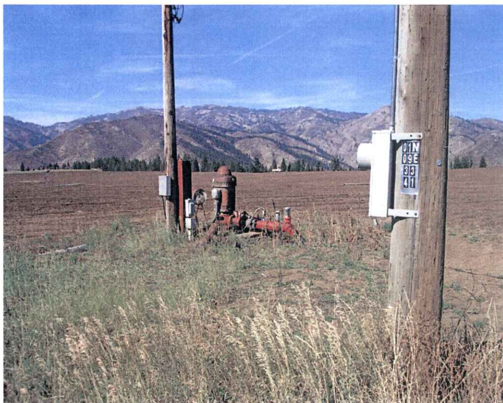
Well #4 – Pole 01N, 09E, 33-41 ( Looking NW )
