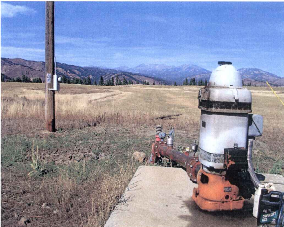
Well #6 – Pole 01N, 09E, 33-11 ( Looking NW )
