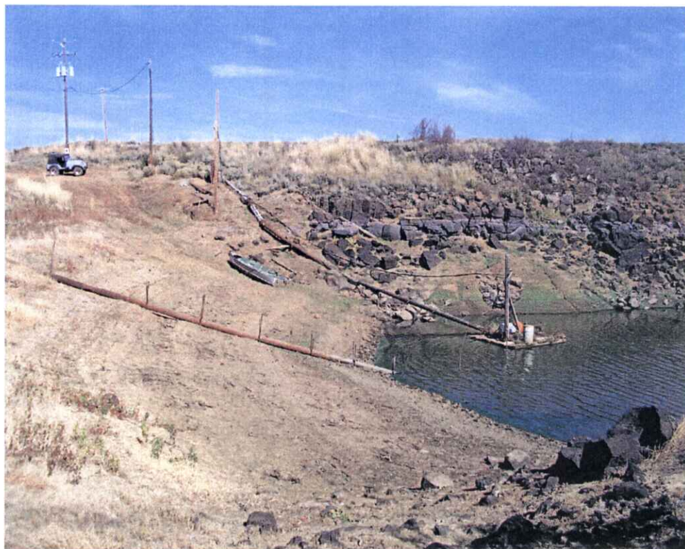
Rhead Reservoir Pumping Plant ( Looking N / NE )
