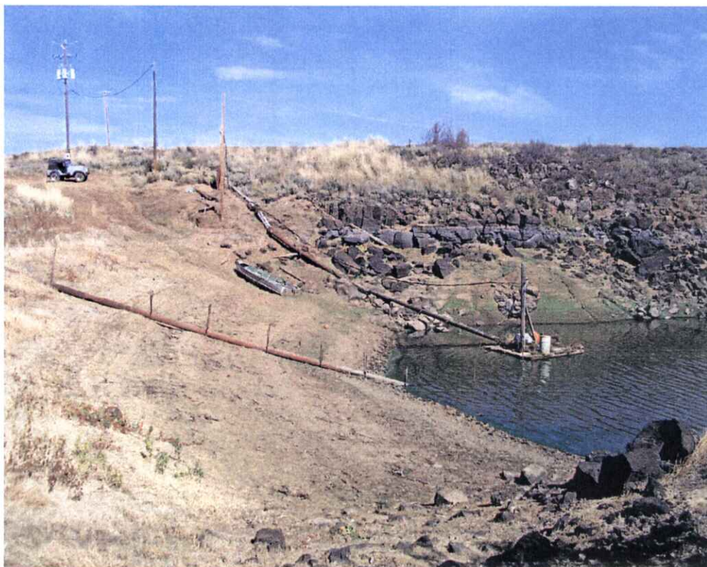
Rhead Reservoir Pumping Plant ( Looking N / NE )
