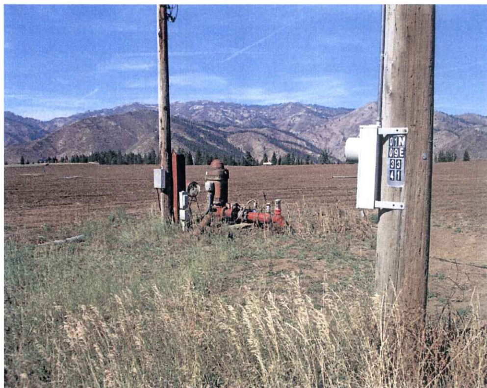
Well #4 – Pole 01N, 09E, 33-41 ( Looking NW )
