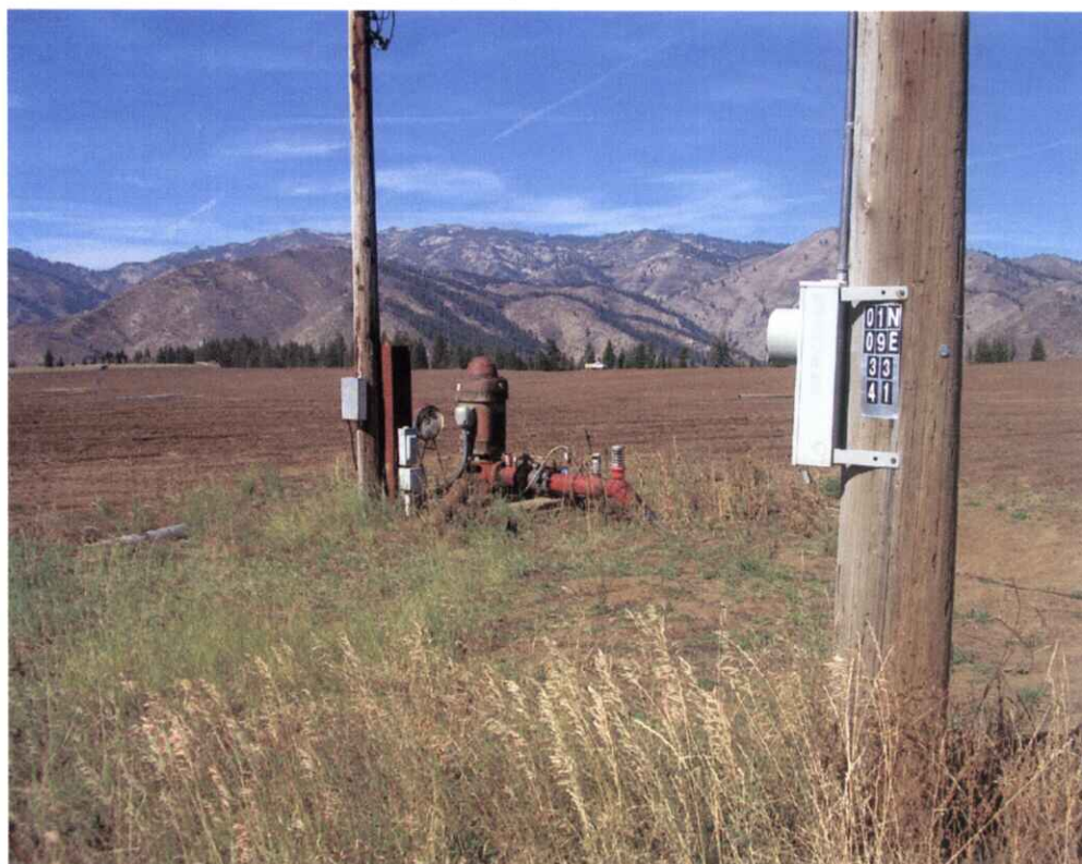
Well #4 – Pole 01N, 09E, 33-41 ( Looking NW )
