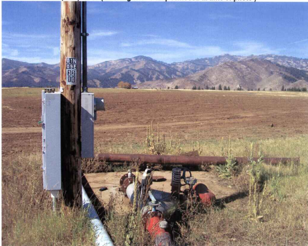
Well #2 – Pole 01N, 09E, 32-10 ( Looking NW - Pump removed at time of photo )
