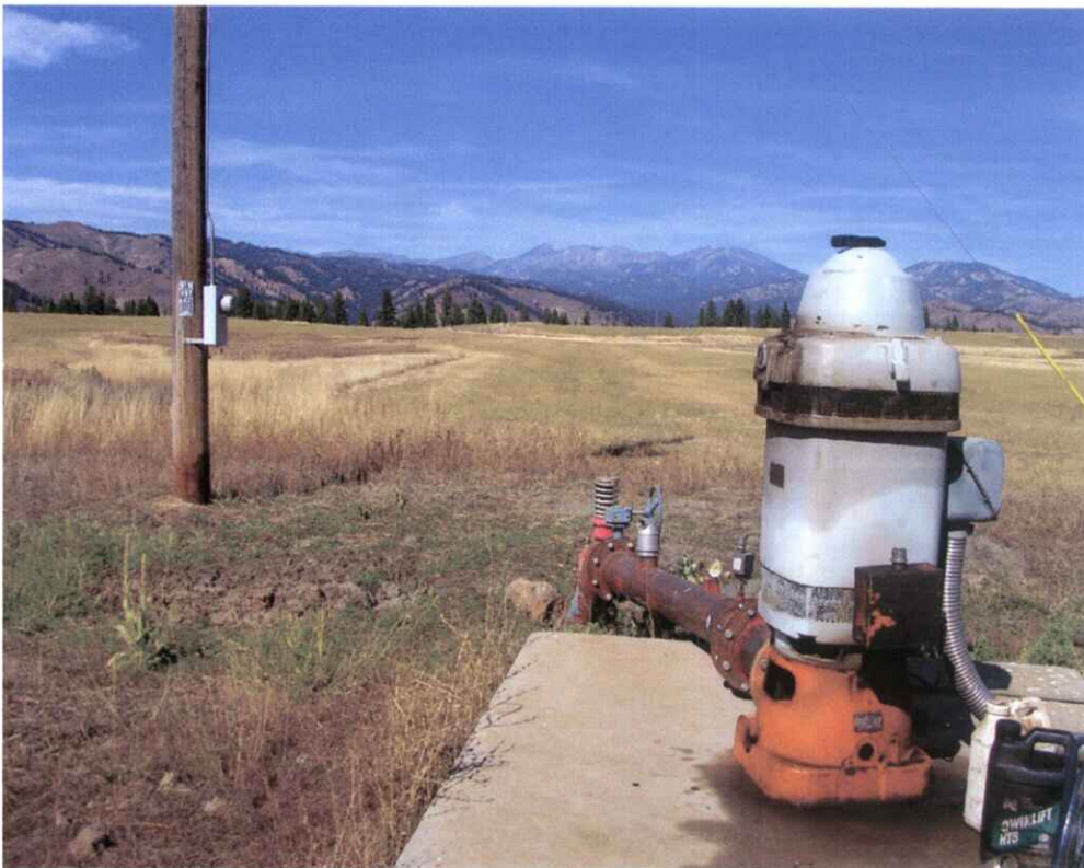
Well #6 – Pole 01N, 09E, 33-11 ( Looking NW )
