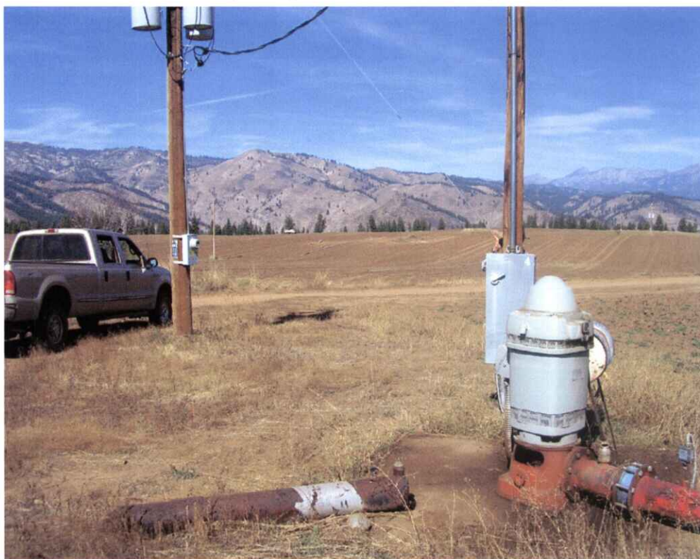
Well #3 – Pole 01N, 09E, 33-40 ( Looking NW. Well #4 shown background right)
