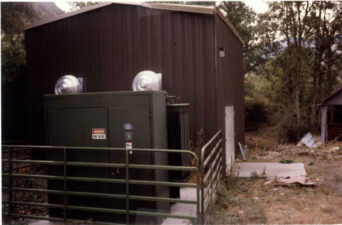
P/W. Powerhouse & Control Panel
