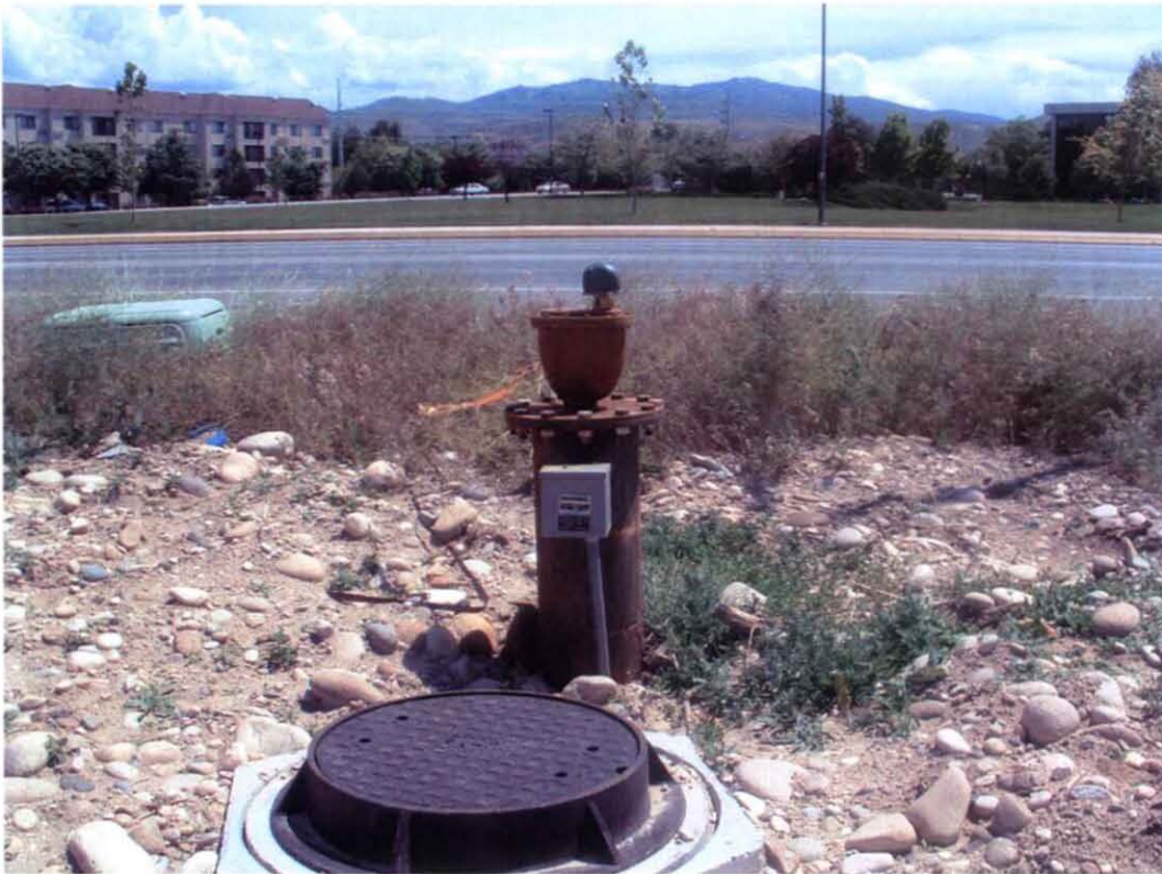
Figure 9. South Injection Well. Air and vacuum valve on top of well. Air release vault in foreground.
