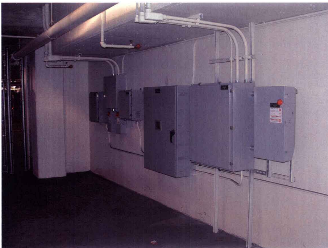
Figure 7. Production well pump controls in basement of Idaho Water Center.
