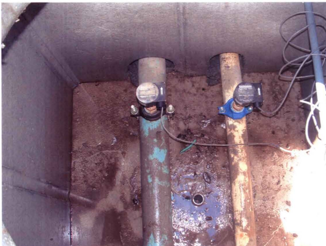
Figure 3. Flow meters for West Production Well pumps in vault.
