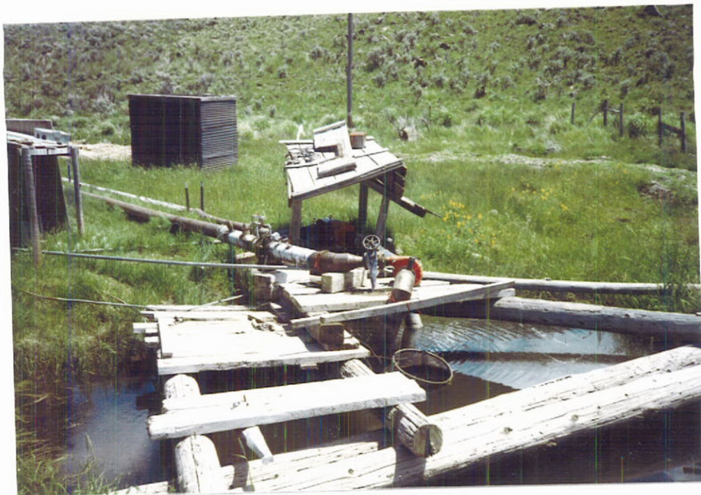
Looking at suction side of Pumps, - 3 ft from W.S to Pump & →
