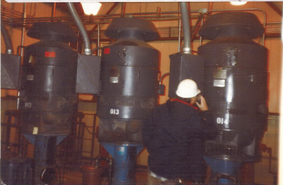
Seepage return Pumps
