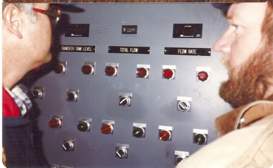
Flow rate & Totalizing readout Panel in Pump House
