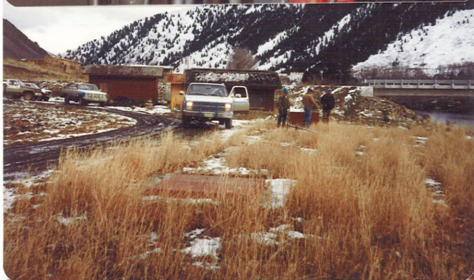
Access doors to sub- surface collectors.
