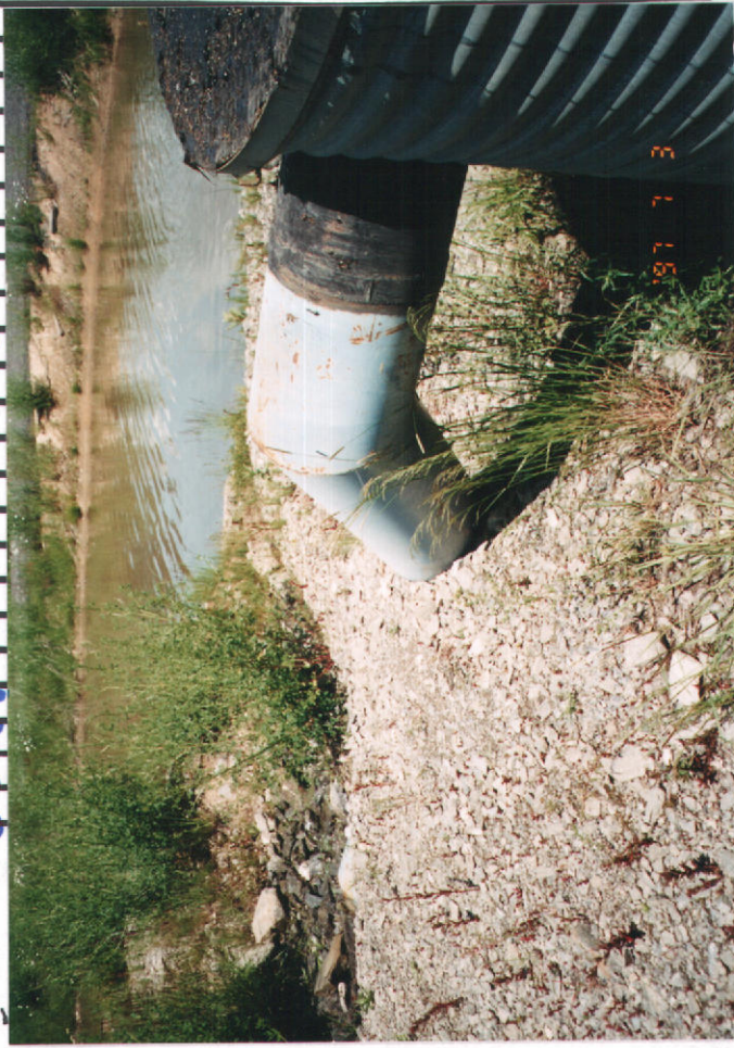
125 HP Vertical Pump overflow from part #2
