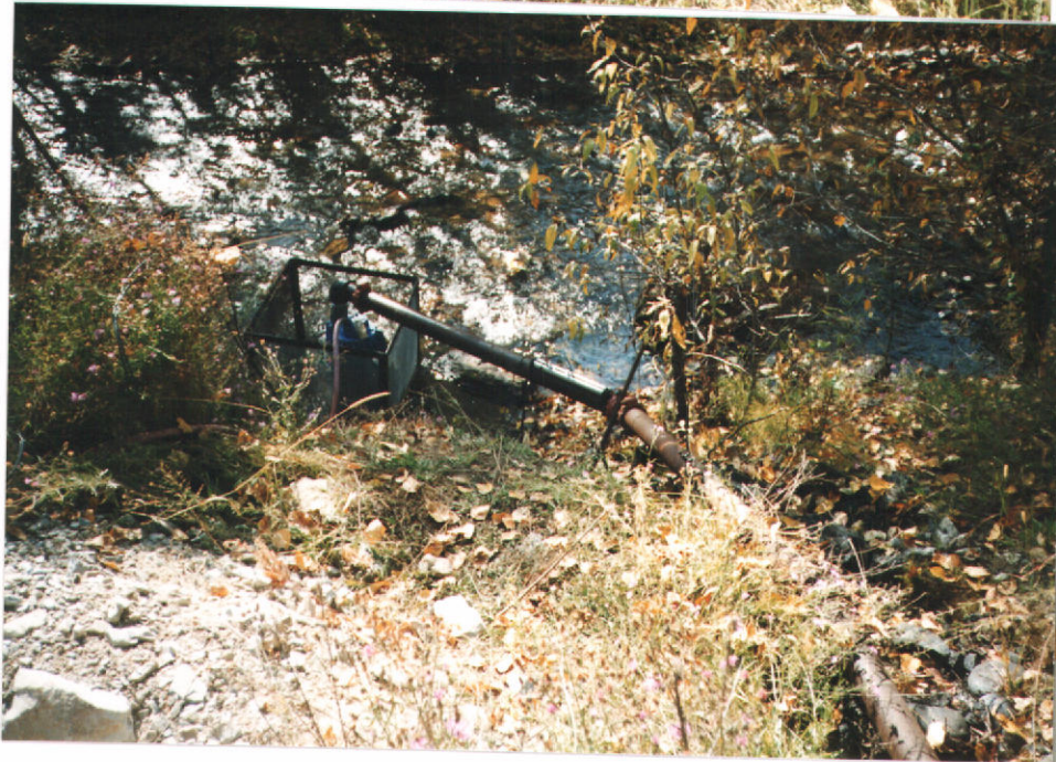
Point of Diversion & Pipeline
