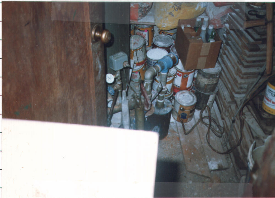
WELL AND WITH BLADDER TANK BEHIND DOOR
