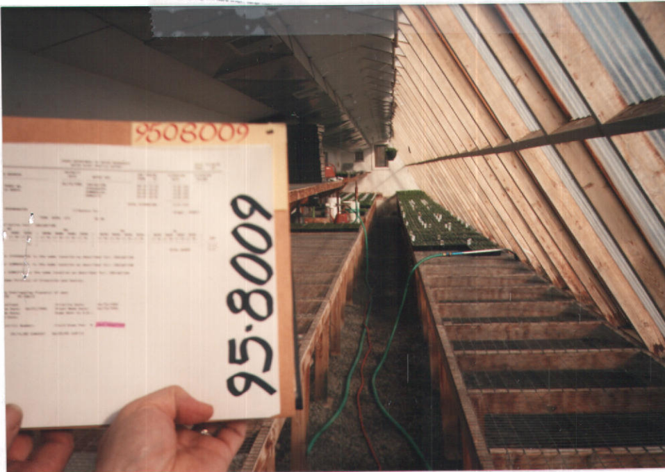
TYPICAL INTERIOR OF GREEN HOUSE
