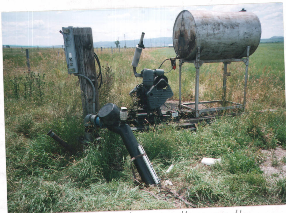
Picture of Generator looking south
