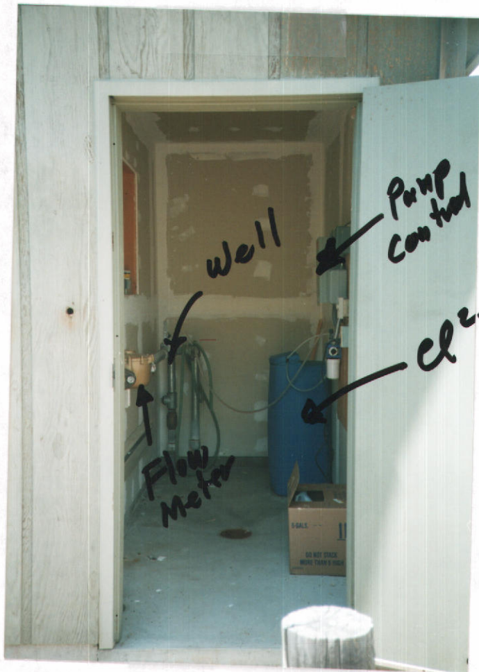
Looking North & West at East side of pump house. show well Flow meter and Cl_2 system
