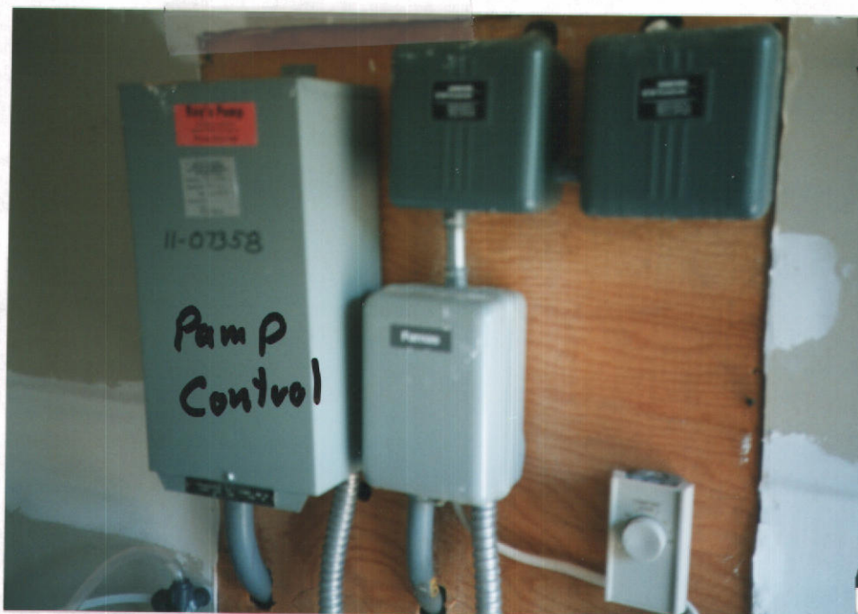
Pump and Cl_2 Control boxes
