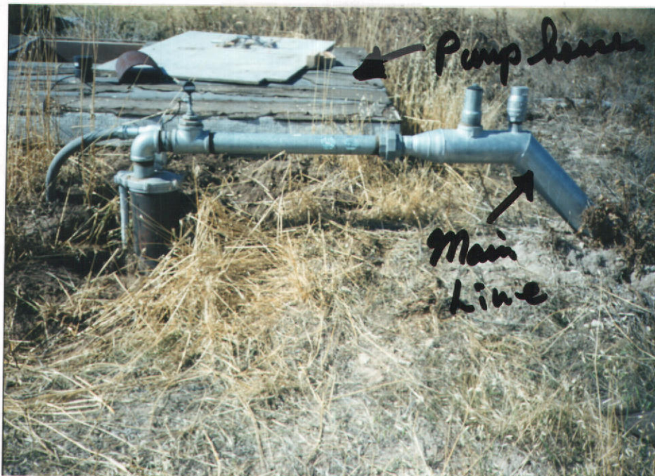
looking South West at well, pump house, and main line connection
