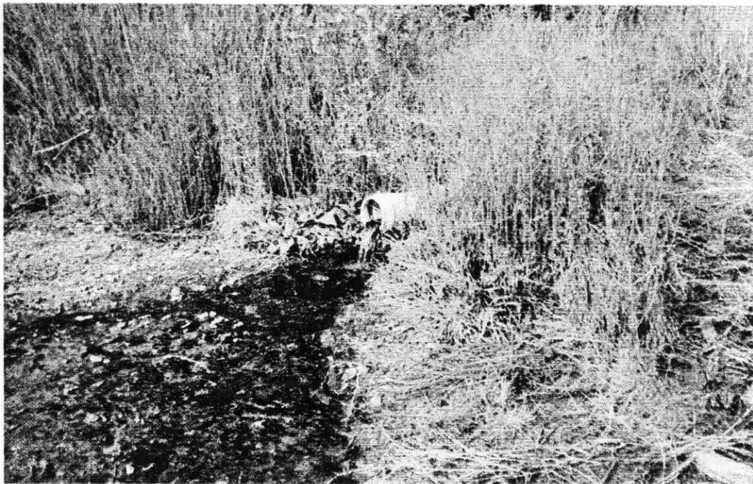
6" Discharge pipe to reservoir @ outfall location
