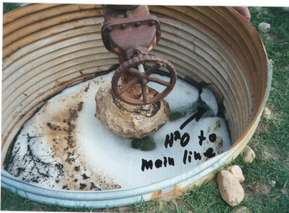
hooking at water entering main line
