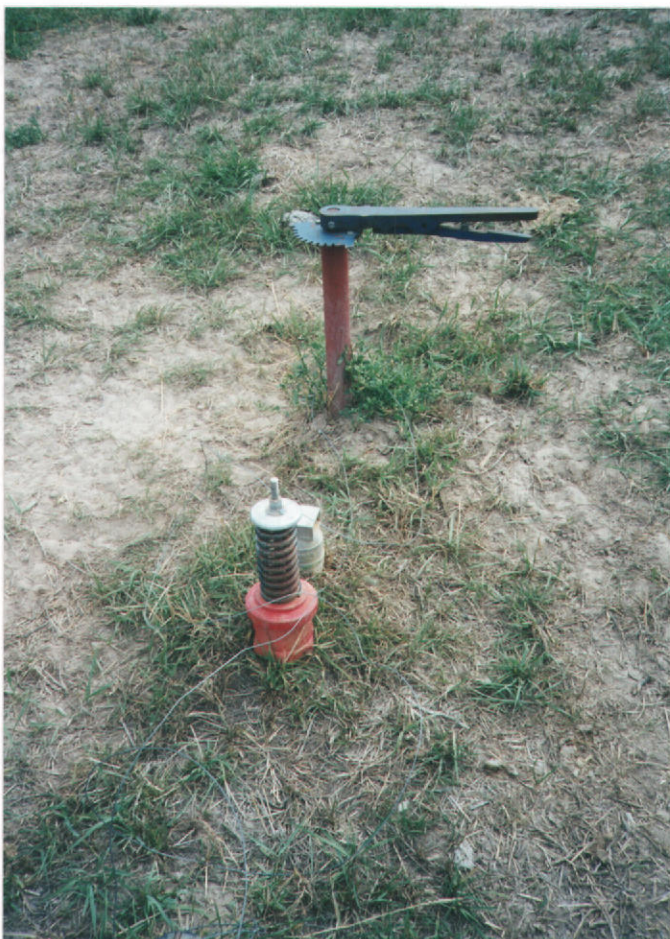
looking at the shut off of the main line in section 20 Note it is closed. looking East
