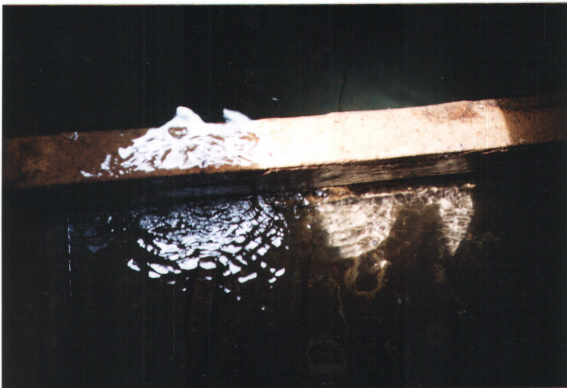
Looking into Collection tank - showing divider - Water from spring enter at top and supply exits at bottom
