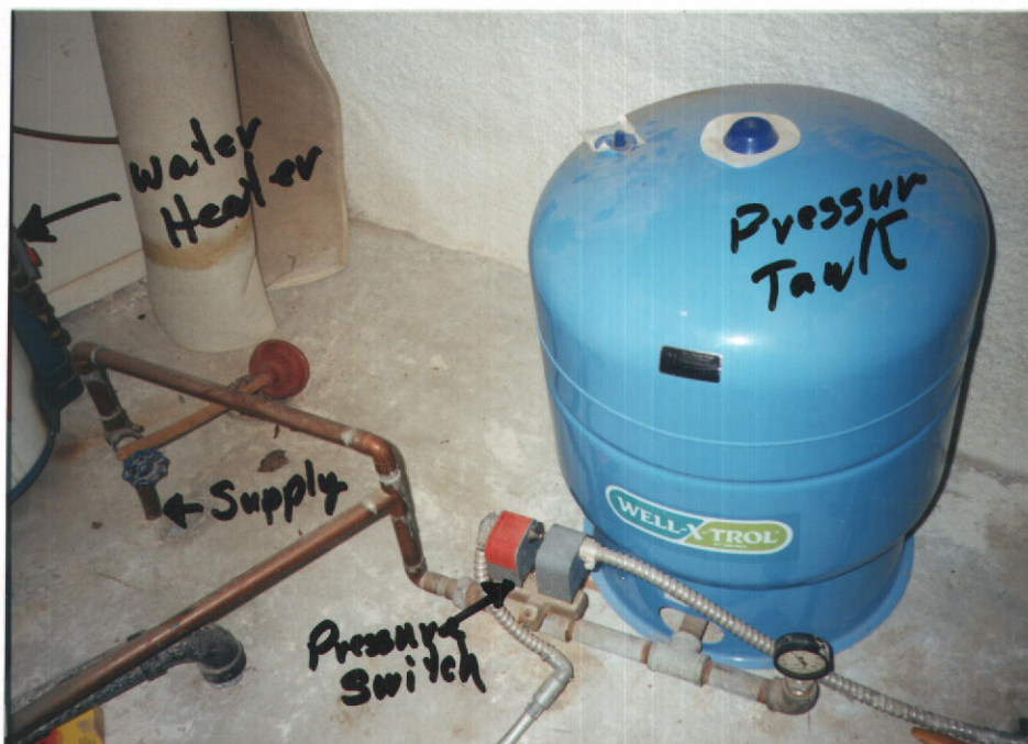
looking at Pressure tank on North side of home
