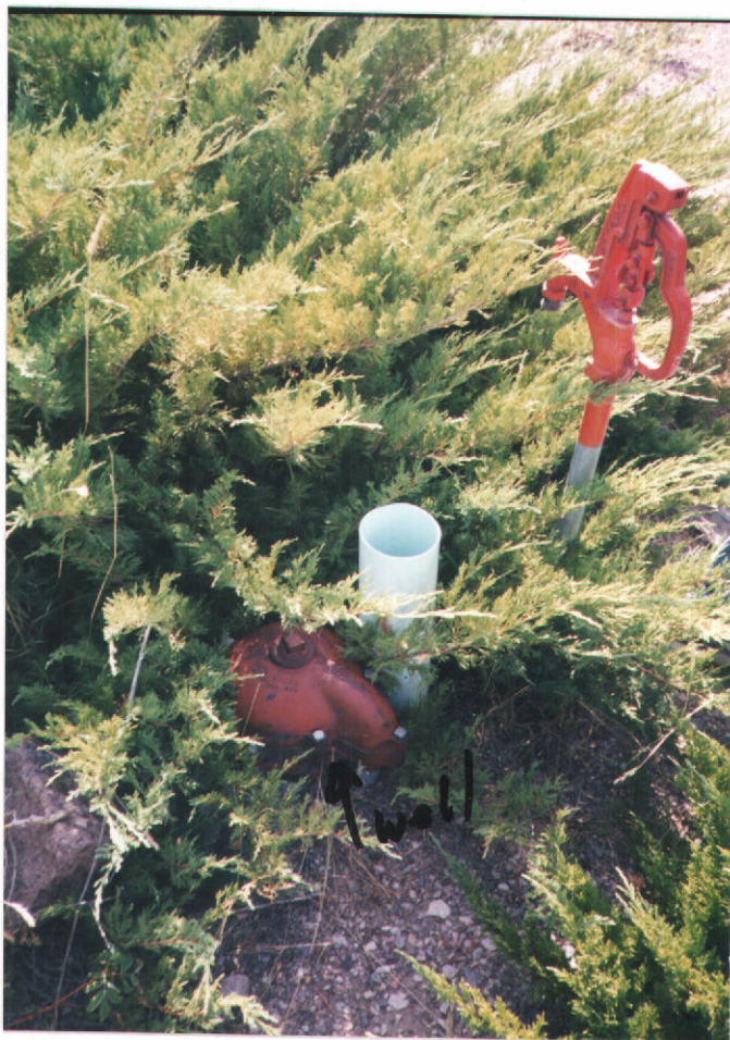
looking South at pump and outside supply
