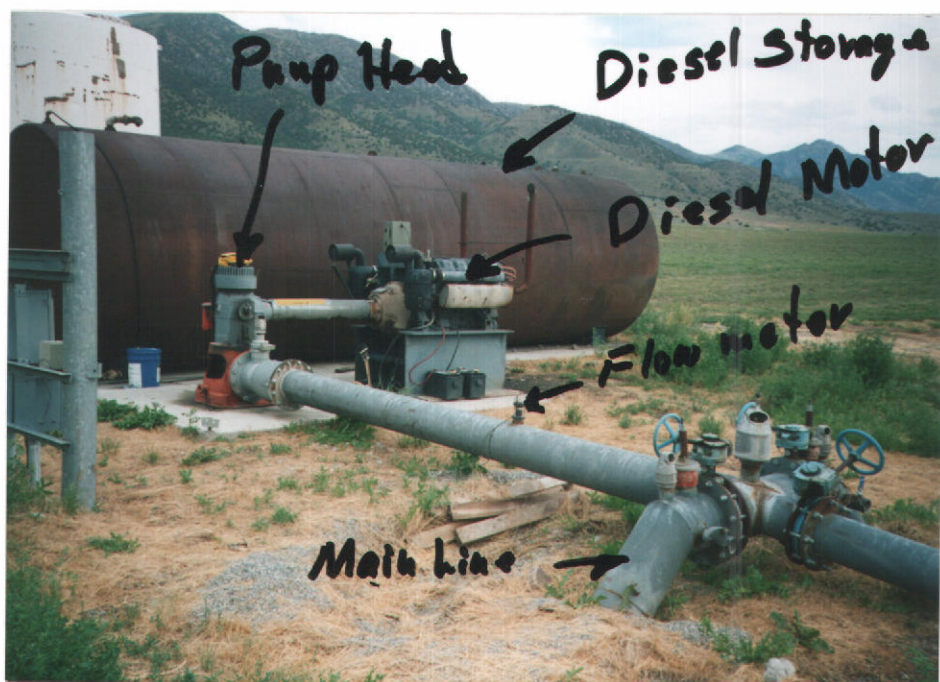
Pump #3 look South East
