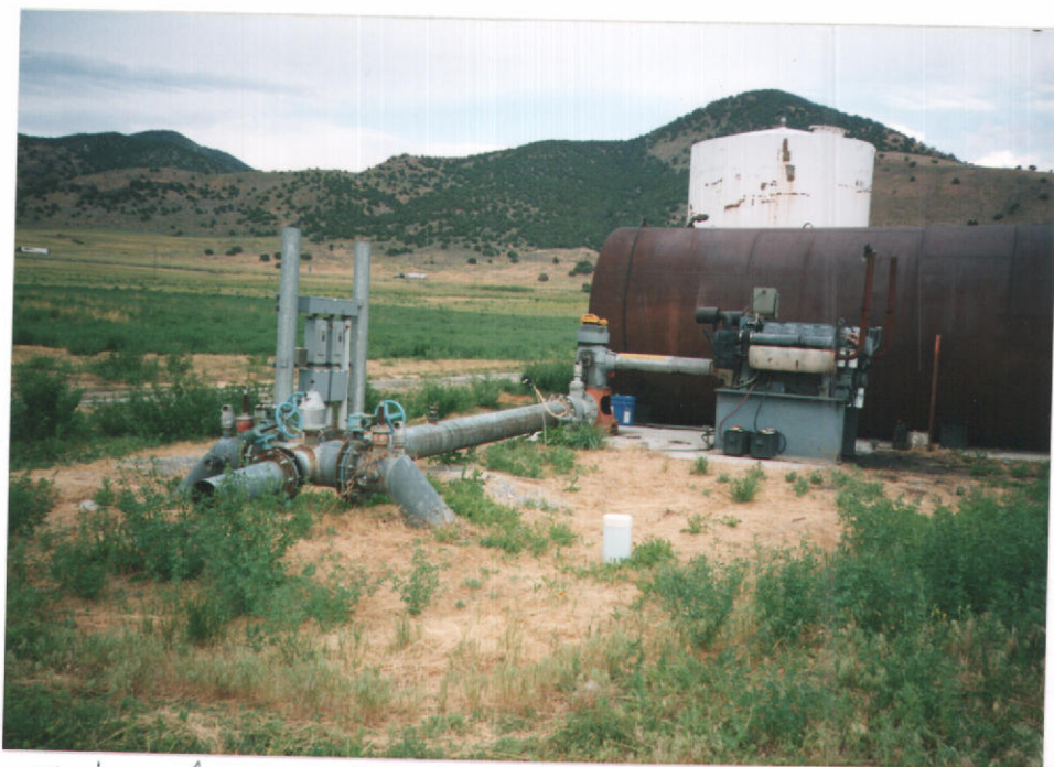
Photo of pump #3 (North) 125 hp diesel look North East
