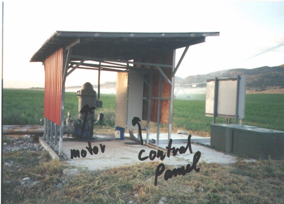
Pump #2 (center) Electric & Control pannel looking North
