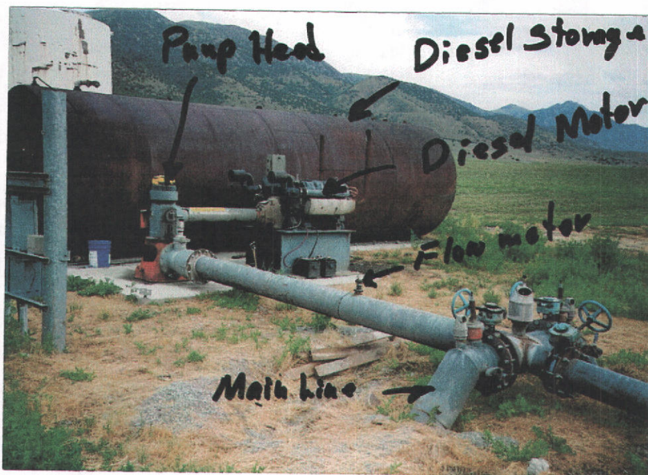
Pump #3 look South East
