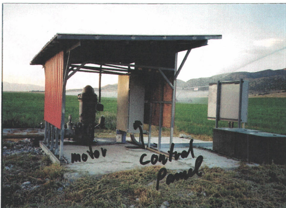
Pump #2 (center) Electric & Control pannel looking North
