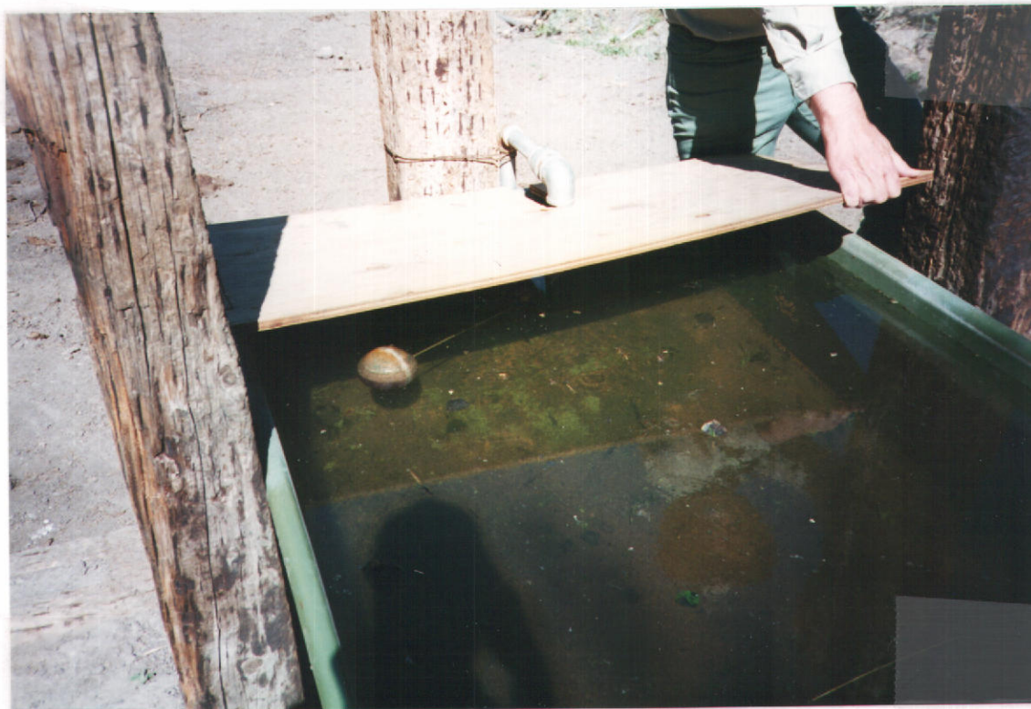
Float Valve on Trough
