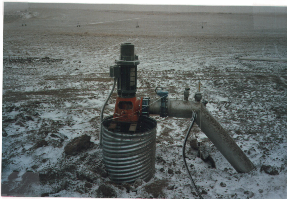
Motor & pump at top edge of Pond
