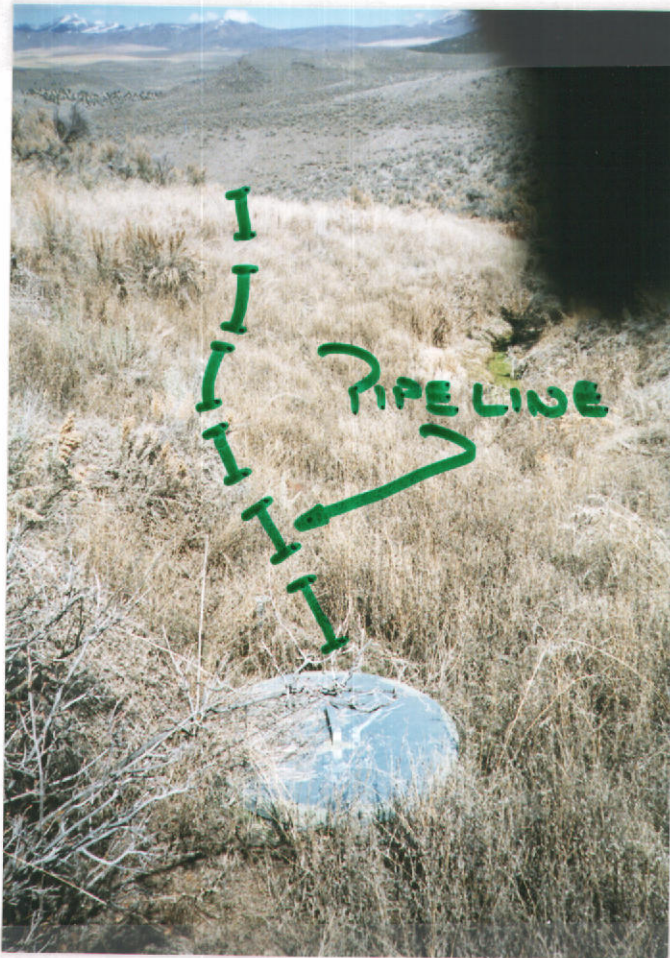
Fig. 1 - Point of diversion valve box and pipeline.
