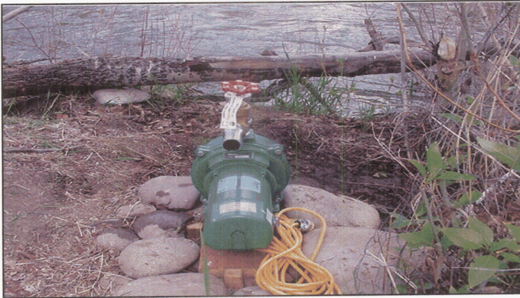
Portable 1 HP Myers Pump. Pump is about 8 feet from the river. The distance from the surface of the river to the ground level is about 30 inches. The river has risen about 1.5 to 2 feet over the past 3 weeks. The pump can be easily removed when the river rises more.
