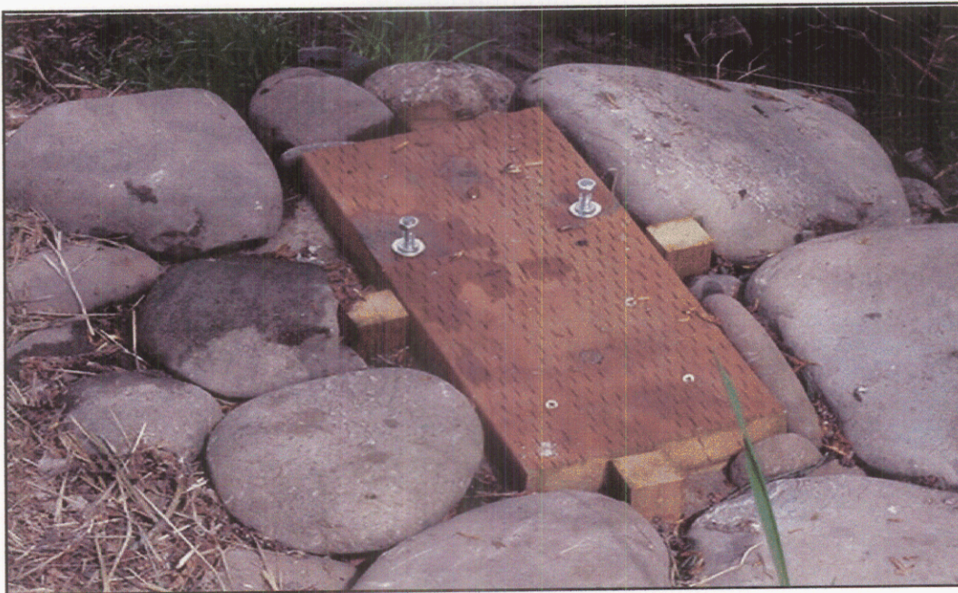
The pump pad is made of 2" X 8" X 16" pressure treated wood (Redwood?). Two of the 2" X 8" X 16" wood cuts have been mounted one to the other with 4" screws. The wood pad is partially buried in the ground. Four stakes secure the wood cuts, with 1 stake on each side of the pad. The pad is shored-up with river rock. 5/16" T NUTS, LOCKS, FLATS and THREAD RODE secure the pump to the pad.
