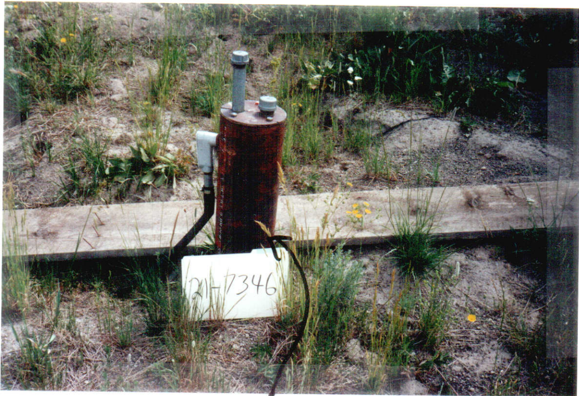
5 HP pump + well location
