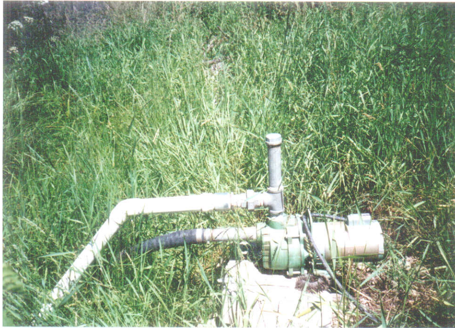
Plate 1 - Point of diversion: Pump #1.
