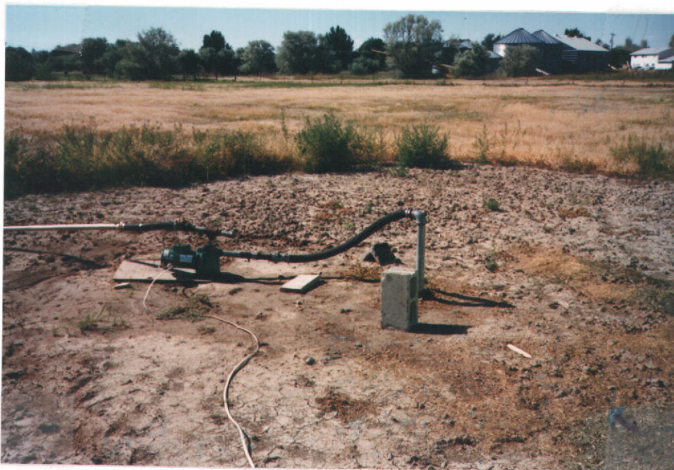
POINT OF DIVERSION #2: DRIVEN SANDPOINT & 5000 GALLON SUBMERGED TANK.
