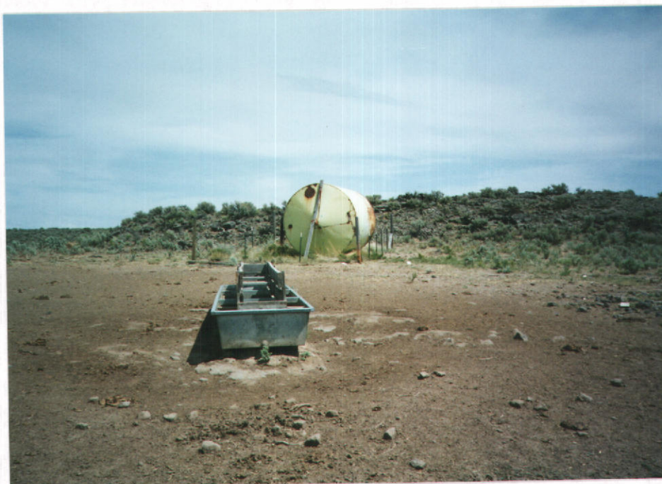
Plate 2 - Complete system showing stockwater trough and 10,000-gallon storage tank.
