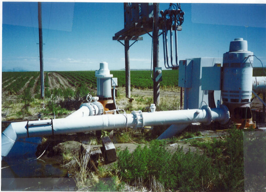
VIEW OF SYSTEM LOOKING NORTH
