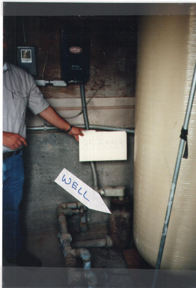
Fig. 1 - Point of diversion inside pumphouse.
