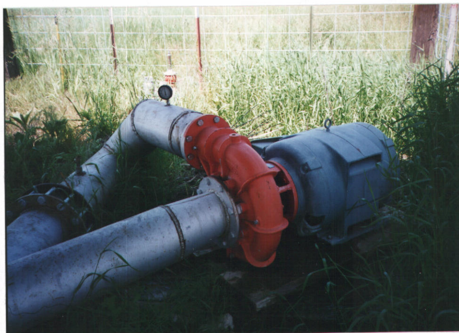
Plate 3 - Closeup of booster pump and motor.
